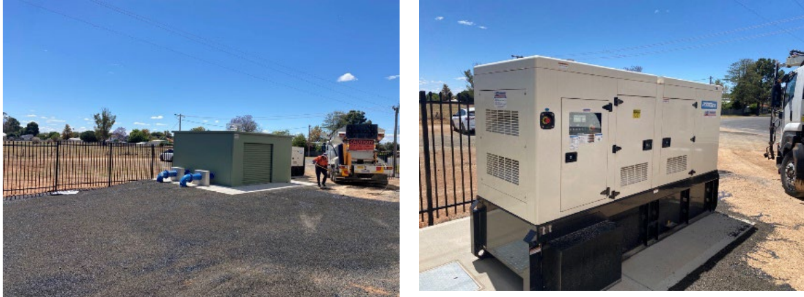
Figure 2: The new booster pump station on Duffy Street, Left: pump station building, right: pump station generator
